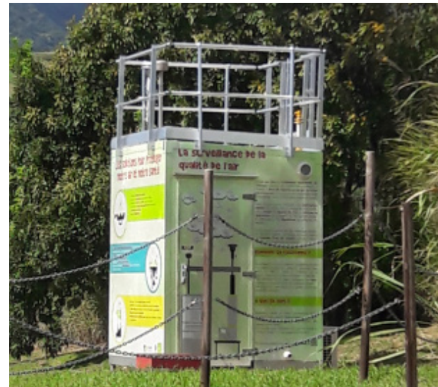
station Saint-Pierre/ CDST
